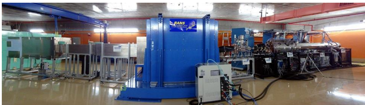
Figure 2: The RANS casemate. (left) scattering instrument (middle) TMR assembly, mostly shielding, (right) accelerator.
