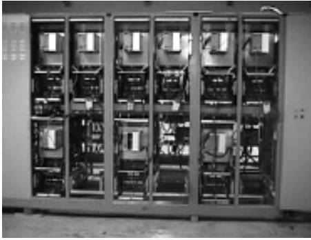
Figure 6. HEXATRONIC implementation: 3000HP @ 4160V power electronic converter.
