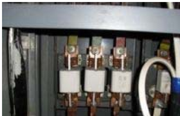
Fig.5. An example of thermal imaging for phase diagnostics in an apparatus of protection and control movement for a mine elevator installation (a photo).
