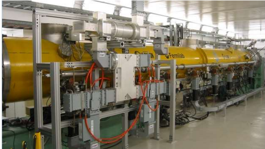
Figure 13: The first 1.3 GHz SRF cryomodule installed in the FAST/IOTA facility.
