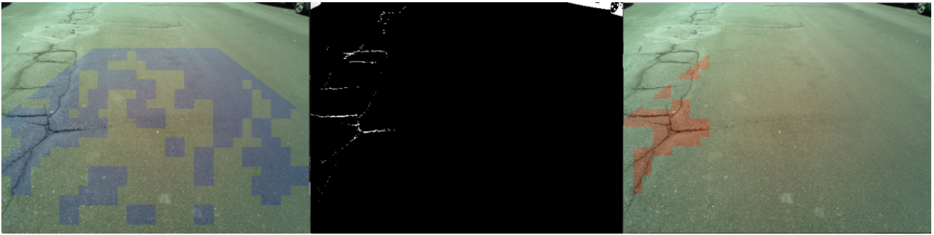
Figure 2: Defect detection result using SVM and adaptive thresholding.
