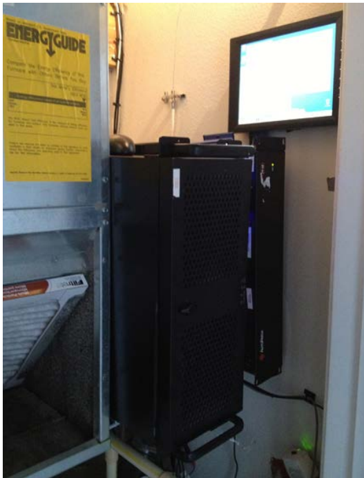
Figure 8. Zac's utility room with HomeSeer server (Cericola, 2013)
