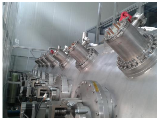
Fig. 9. Gas tank installation for the magnet
