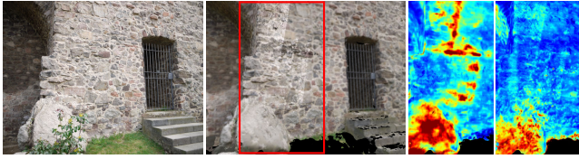
Fig. 10. Left to right : Photo, rephoto with color defect framed in red, 1-NCC and C_b+C_r error projection of the framed segment.
