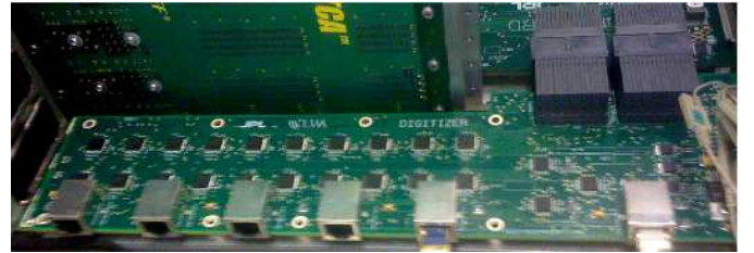
Fig. 10. One of the 26 digitizer boards contained in the DP rack. Each board digitizes 20 antennas, and plugs into a DP1 board (see Figure 11). Courtesy JPL.
