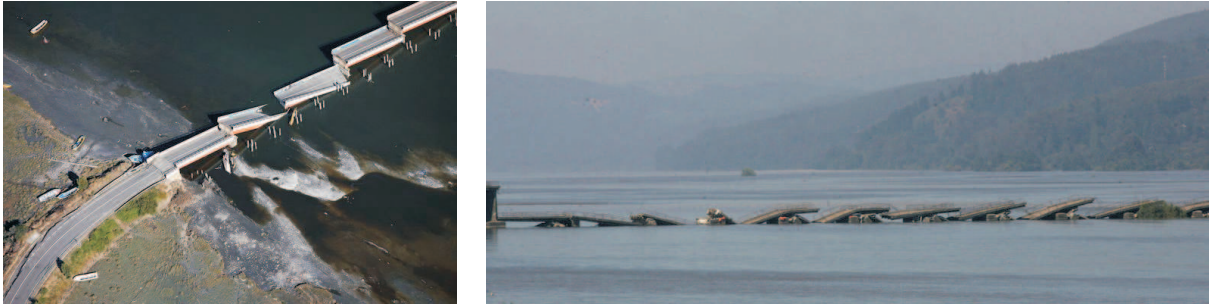
Figure 2: View of the destroyed “Puente Viejo” over the Biobio river, that links Concepcion and San Pedro de la Paz, 500 km south of Santiago, Chile, after the 8.8 magnitude earthquake on February 27, 2010. © Nicolás Piwonka, National Geographic.
