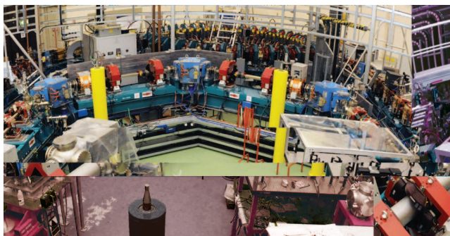
Figure 3: (Colour) Moving TBA arc as installed on ALICE at Daresbury Laboratory. The three blue dipoles each lie over linear bearings upon which the entire arc moves, mounted on a single angled girder.
