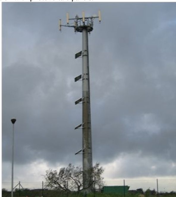
Figure 6. A Photovoltaic installation over a BTS.
