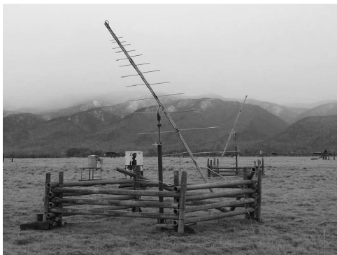
Fig. 5. View of the radio antennas
