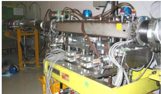
FIG. 3: The installation of the prototype LHC collimator in the SPS tunnel. The figure is taken from [22].
