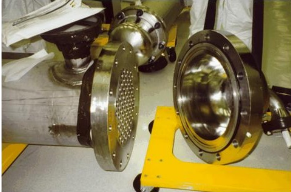
Figure 8. Close up view of the double gasketing system on flanges for leak tightness. The double gasketing system was employed throughout the purification skids. The outer gasket is a teflon encapsulated viton O-ring. The inner gasket is a metal helicoflex™ gasket. The mirror finish of the electropolished stainless steel used throughout the purification system is also evident.
