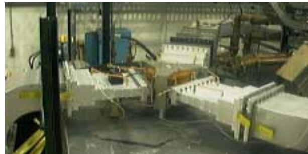
Figure 4: Atlantic Microwave 700 MHz 100 kW Circulator Installed on the Test Stand.
