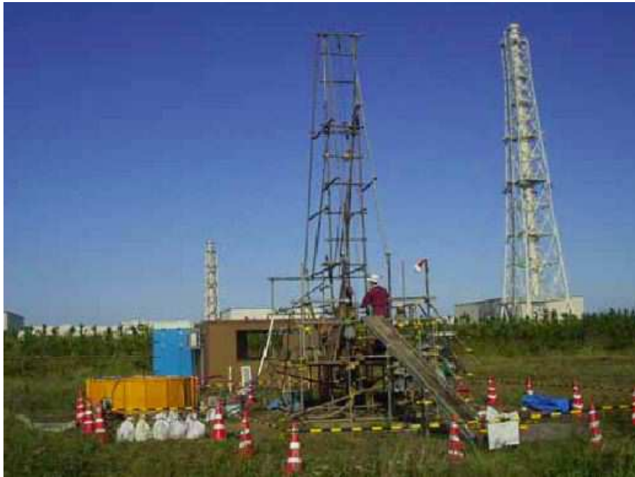
Figure 43: Boring study at the near-B site. The towers behind the boring scaffold are ventilation towers of reactor buildings.
