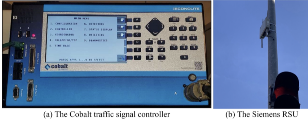
FIGURE 5 Signal Controller and RSU (23)
