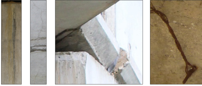
Figure 22: Bridge structural concrete images adapted from the CODEBRIM dataset [Mundt et al., 2019] under its specific license. From left to right, as named in the original dataset: 1) image_0000005_crop_0000001.png - contains efflorescence and corrosion stain defects. 2) image_0000046_crop_0000001.png - contains crack defects. 3) image_0000109_crop_0000003.png - contains spallations and corrosion strain defects. 4) image_0001189_crop_0000004.png - contains exposed bar defects.
