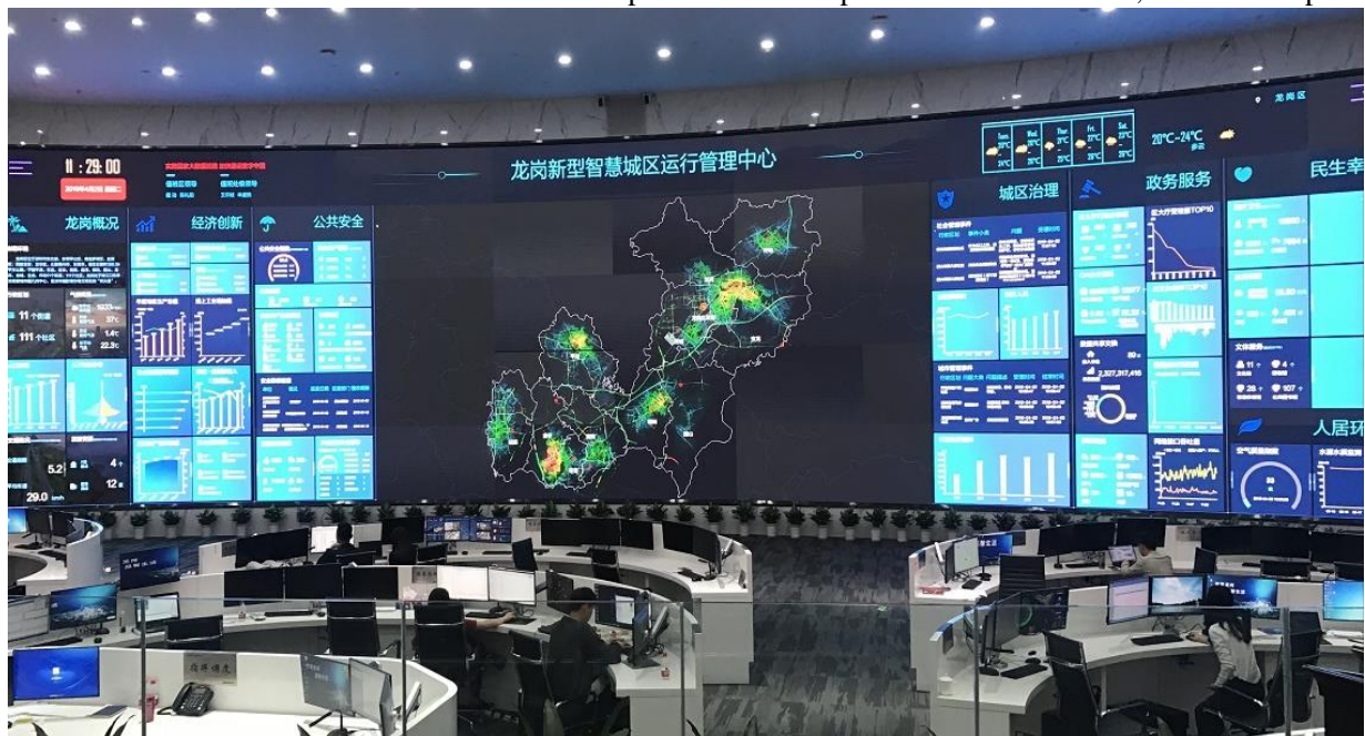
Fig. 3 The LED screen at the Longgang Smart Center
