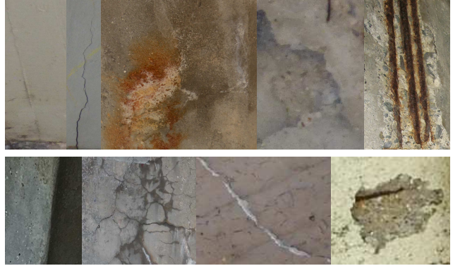
Figure 1. Example damages from CODEBRIM (top line) and MCDS (bottom line). The labels for CODEBRIM are No Damage, Crack, Efflorescence/Rust, Spalling, Spalling/Exposed Bars/Rust. The labels for MCDS are No Damage, Crack, Efflorescence, Spalling/Exposed Bars/Rust.
