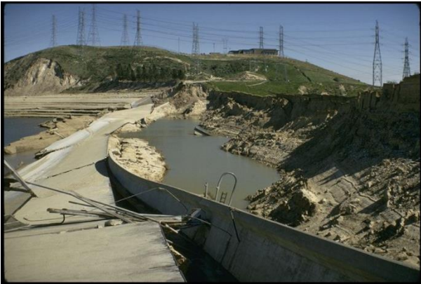
Figure 2. Side view of the Lower San Fernando Dam (Steinburgge Collection, 1971; NICEE Library, University of California Berkeley; after Chowdhury, 2019).
