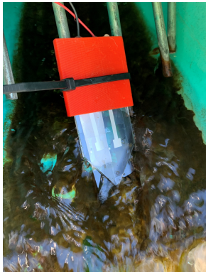
Fig. 5: Nitrate sensor of a sensor node in a farm drain tile. A tile drainage system consisting of a network of underground pipes allowing subsurface water to move out from between soil particles into the tile line.
