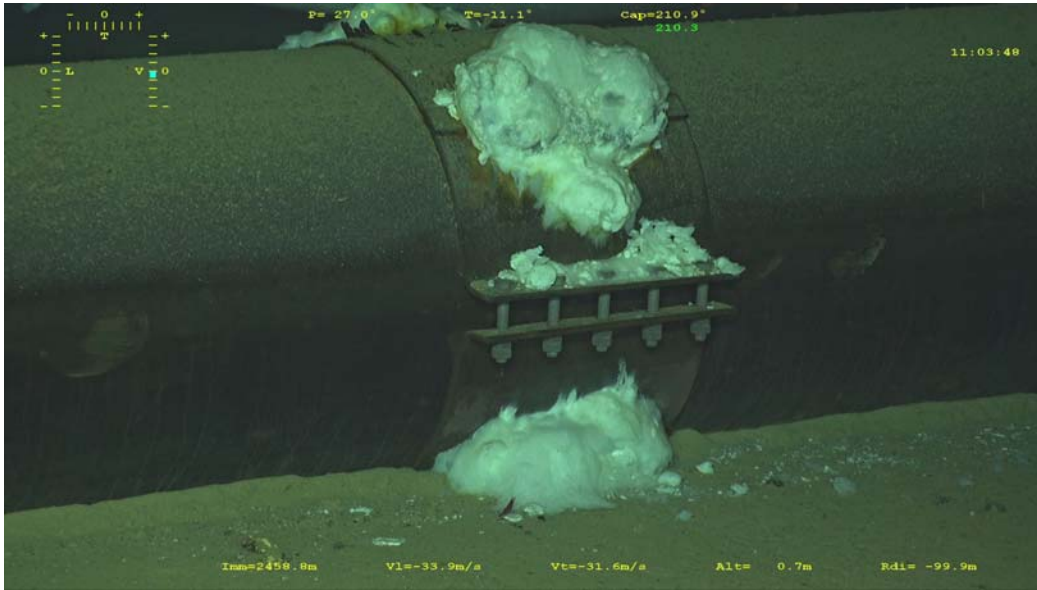
FIG. 14. Detail of cable attachment saddle with heavily deteriorating zinc-aluminum-alloy anode.
