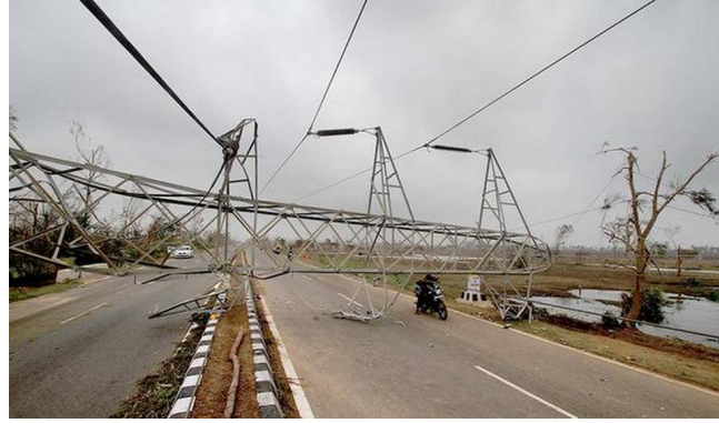
Fig. 1. A collapsed tower in Puri district of Odisha during 2019 cyclone Fani (Photo Credit: Biswaranjan Rout; taken from www.thehindu.com , accessed March 10, 2020).
