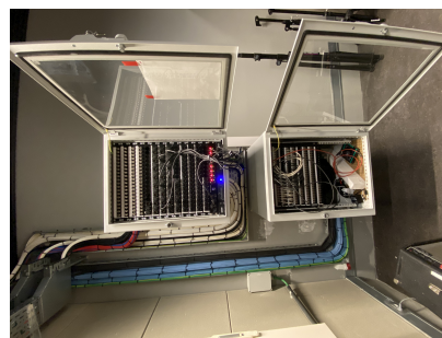
(b) Patch Rack
