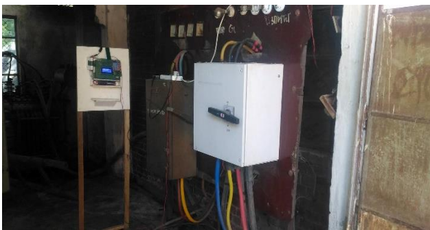
Fig. 7. Implementation in Mirpur Cantonment area switching station
