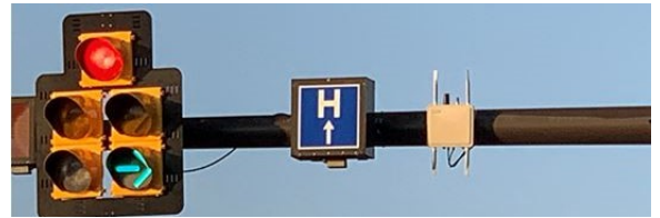
Fig. 10: The roadside unit at the intersection. Photographed by City of Dublin [29].
