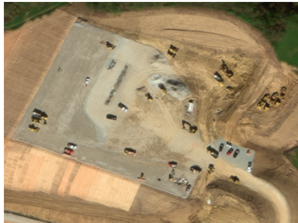
Fig. 1. This is an example of a fracking well during the construction phase. The ground has been excavated and the rock formation is being laid down to form the well pad. Image: DigitalGlobe, Inc.
