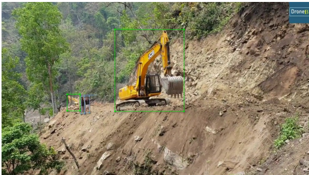
FIGURE 6. Four objects can be clearly seen in the image; even the excavator in the distance is much smaller than the one nearby. Moreover, the two standing workers can be recognized as well.
