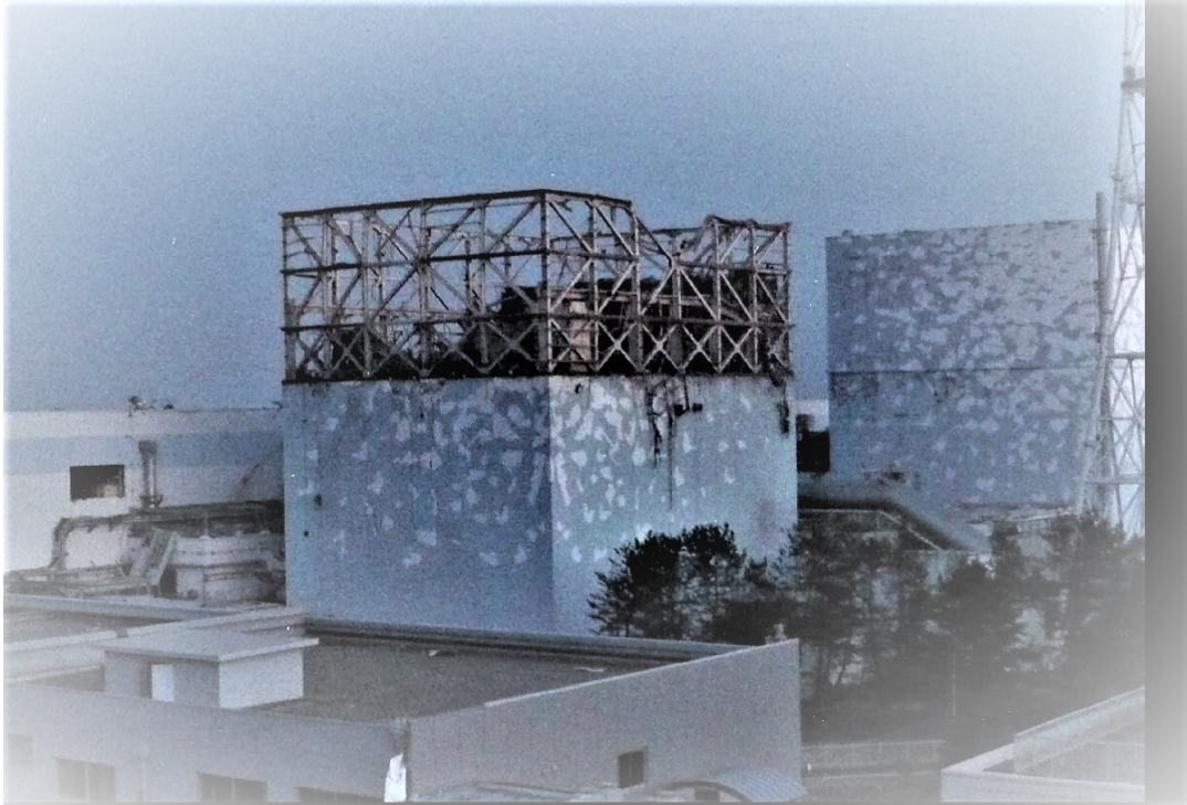
Fig. 1. Damaged Unit-1 Reactor of the Fukushima-Daiichi, viewed from north-west side. The Unit-2 building is seen to the right. (Courtesy of TEPCO).
