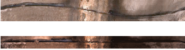
Figure 8: Detail views for the pipe couplings (cropped and rotated from Figure 6 ). Top: Typical artifact due to an incorrect camera pose estimation by the commercial sewer pipe inspection software. Bottom: The distortion free pipe coupling as a result of the camera pose estimation.
