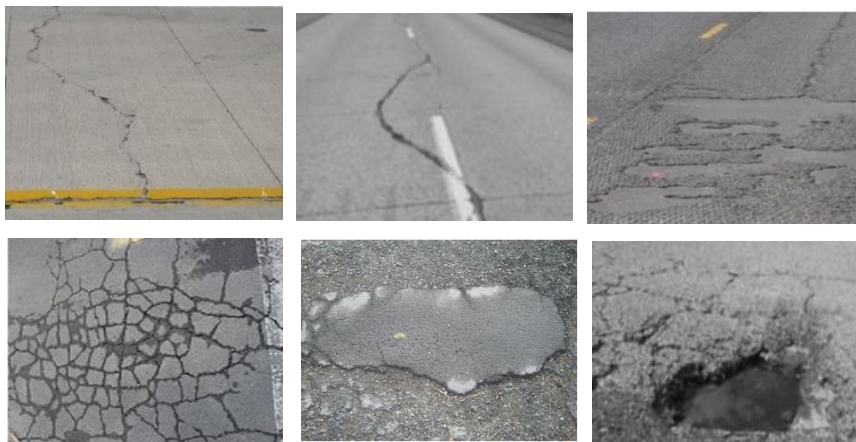
Fig. 1. Examples of structural damages typically found in the literature: a-b) linear cracks, c) peeling, d) alligator cracks, e) patches and f) potholes
