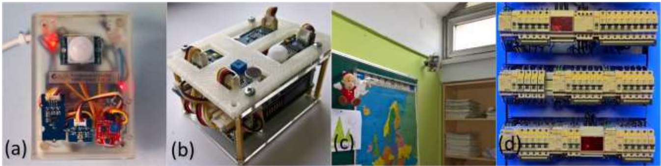
Figure 1. Sample photos of the device lineup inside GAIA's schools: a) an Arduino-based IoT node for classrooms, b) a Raspberry Pi-based node for classrooms, c) an IoT node inside a classroom, d) power meters installed on electricity distribution panels.
