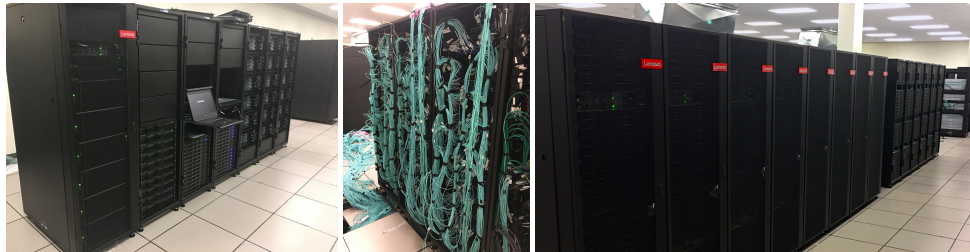
Figure 1: SciNet's Niagara supercomputer at the University of Toronto. From left to right: management nodes, Dragonfly interconnect, racks with compute nodes.
