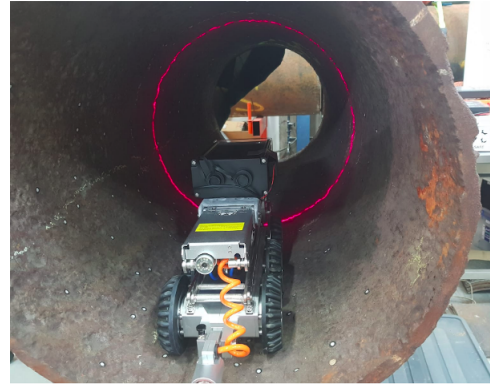
Fig. 7: The robot scanning a corroded metal pipe. Red laser projection has been used instead of the IR laser for image demonstration purposes.
