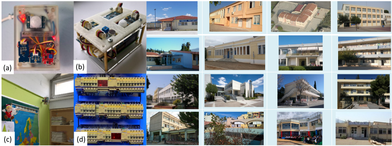
Fig. 1. Examples of the IoT infrastructure located inside school buildings in Greece (a-b) IoT nodes based on Arduino and Raspberry Pi, c) actual node inside a classroom, d) a power meter installed inside a distribution board at a Greek school, along with photos from the exterior of some of the school buildings.
