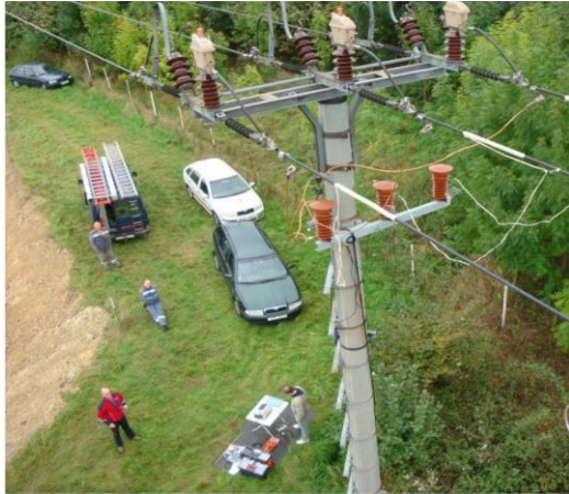
(b) Coils connected to three phases of a medium-voltage power line
