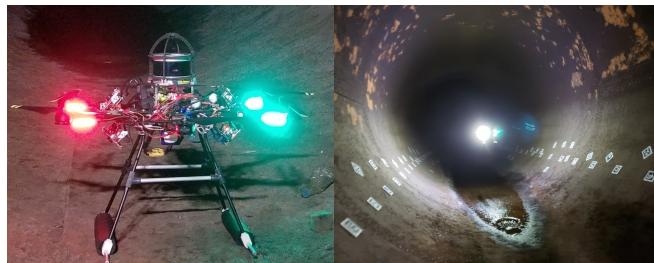
Fig. 1: The MAV platform flying inside a penstock at Center Hill Dam, TN. The robot collects images from four on-board cameras with the only illumination source being the on-board power LEDs.
