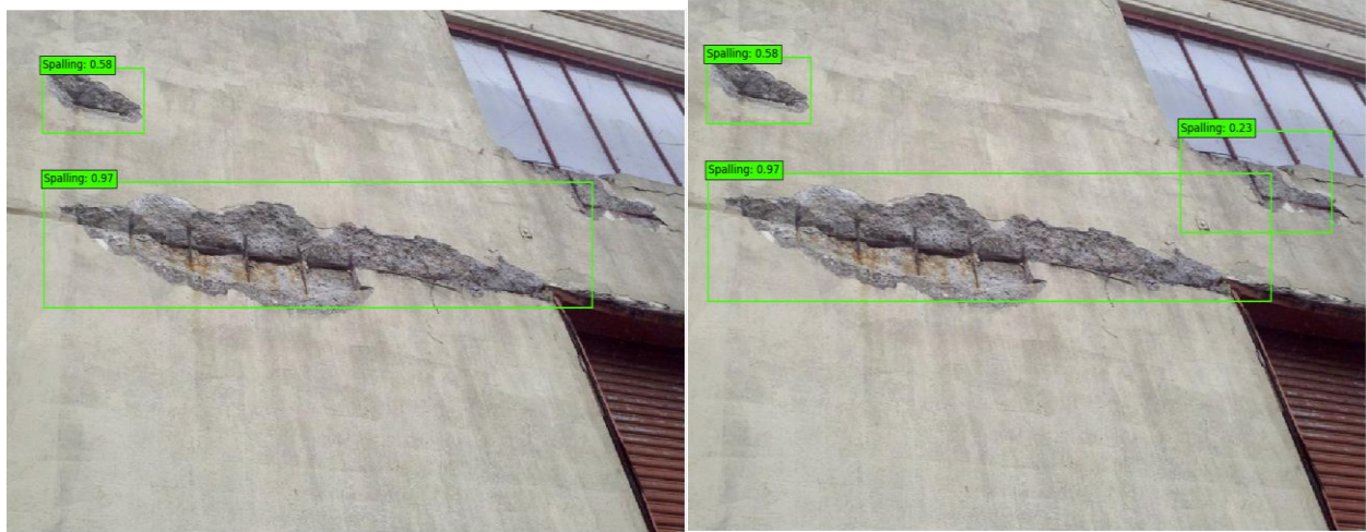
Figure 10 Example of human-AI collaboration in the proposed methodology (detection AI alone on the left misses a spall, while human-assisted AI detects all spalls on the right with threshold adjustment by the inspector).
