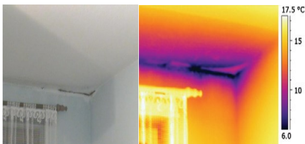
Figure 13: Validation of a potential damage to a structure due to water leakage through visual IR imaging
