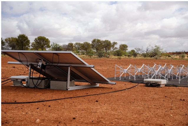
Figure 4. A Phase II long baseline tile. The batteries and beam-former interface systems are located under the solar panels.
