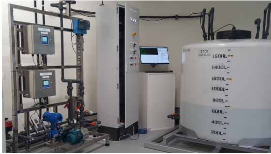
Fig. 6: Process P1 (raw water treatment) – SWaT testbed
