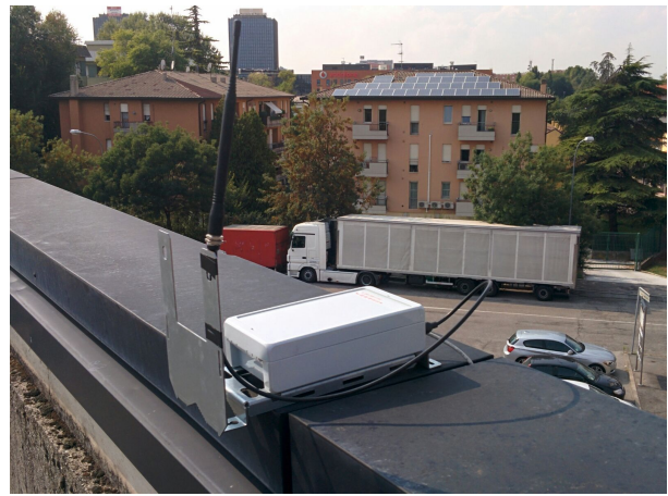
Fig. 3: LoRa™ gateway installation.
