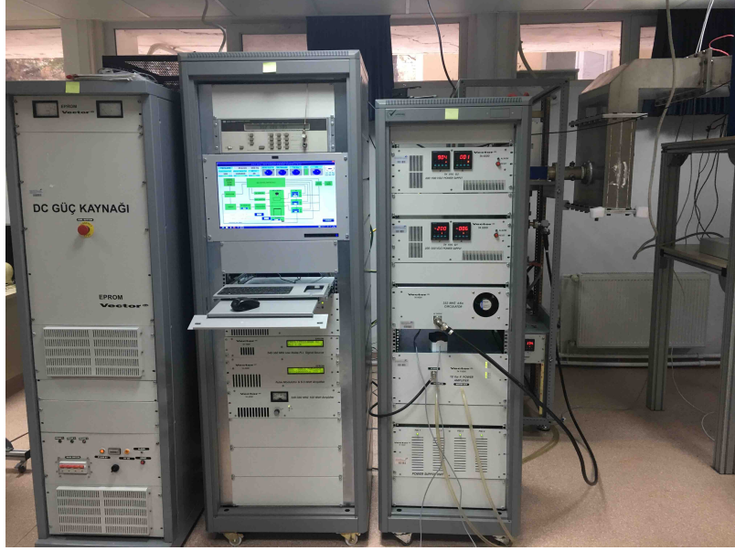
Figure 8. SPP PSU in use. The left rack has the DC power supply, the central rack has the controller and the master signal generator, and the right rack has the power supplies for the tetrode gates, the first amplification stage and the output to the Tetrode amplifier rack.
