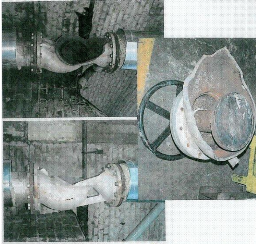
Figure 1: Examples of pipeline damage caused by water hammer (Source: http://traction.armintl.com/traction#/single&proj=Docs&rec=403&brief=n )
