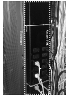
Fig. 3. Smart-PDUs deployment at MEF data center
