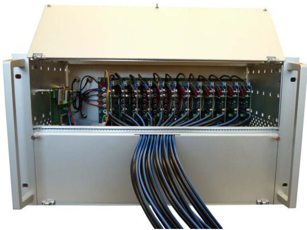
Figure 6. The MAWG device showing the control-board (on left) and the backplane housing 12 daughter cards on it.
