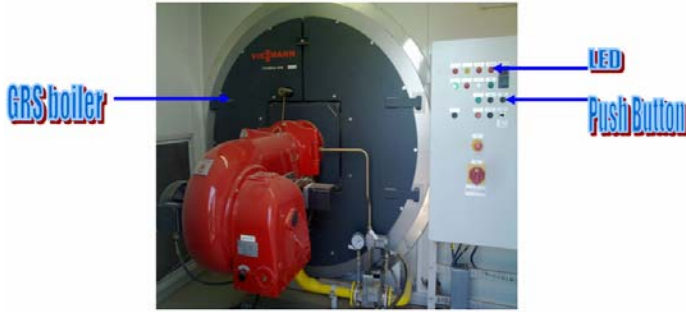
Figure 2. Local control panel of GRS
