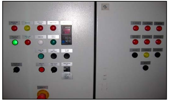
Figure 21. Response of GUI in case of “circulation pump” Figure 22. Response of Local Panel in case of “circulation pump”
