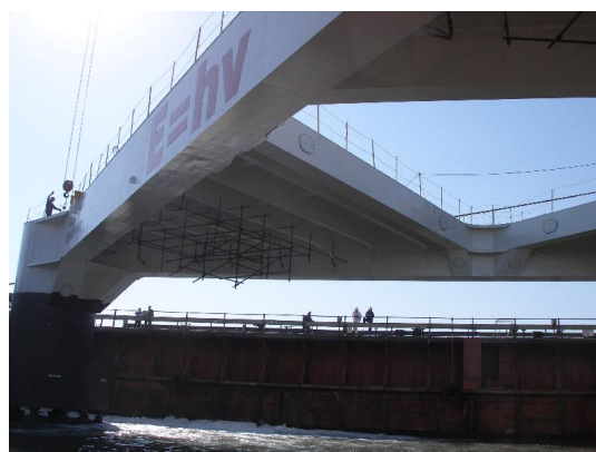
Figure 24. Photograph of the Delta Berenike platform in the final phase of its construction.
